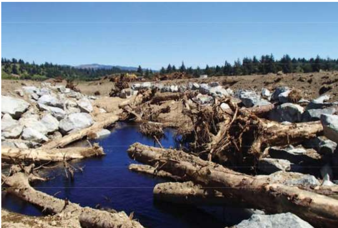
Fish passage-grade control rock structure. The rock features in the lower end of the alignment (pool-riffle) will be below groundwater, but they were designed and constructed to withstand southward migration of the Sixes River channel, which would change the overall slope of the lower Sullivan Gulch channel. Photo credit: Curry Watersheds Partnership.
