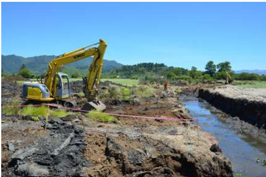
Removing dikes to reconnect the floodplain with the river, creating tidal channels that provide rearing habitat for salmonids, and planting native species to restore spruce swamp wetlands are key goals of the Kilchis restoration project. Photo credit: The Nature Conservancy.
